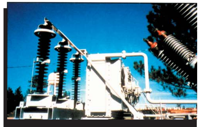
Proximity of high voltage arresters to forced-oil radiators and high voltage bushings was of great concern.
