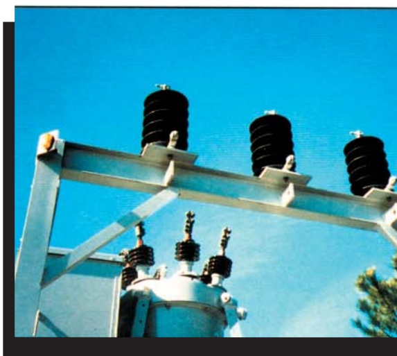
New 21kV PVN arresters.
