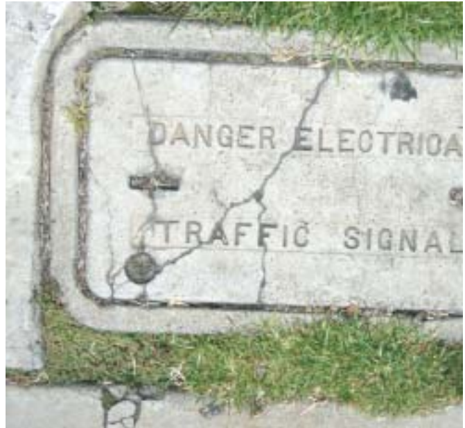
A cracked cover is a failed cover because its design performance capability has been compromised.
