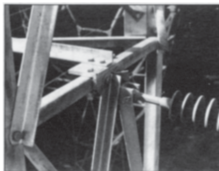
Tower attachment of phase-ground insulator
