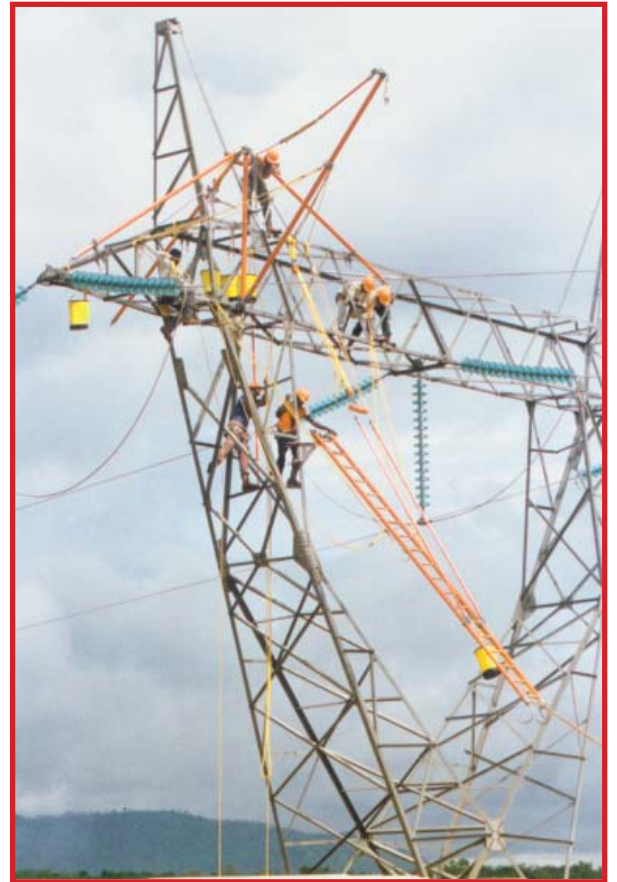
Tanzania, above, crew raises hook ladder while learning cargo-boom method for live installation of deadend insulators on 230 kV free-standing tower.
