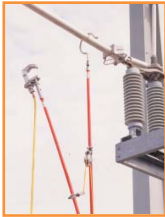
Teamwork safely lands the large clamps required to ground substation buswork. Shepherd-hook assist stick features a sheave with lift line to manage control.
