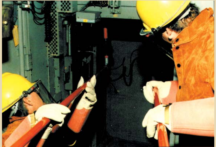
Plant electricians use Chance phasing tool to confirm absence of line voltage prior to applying grounding cables.
