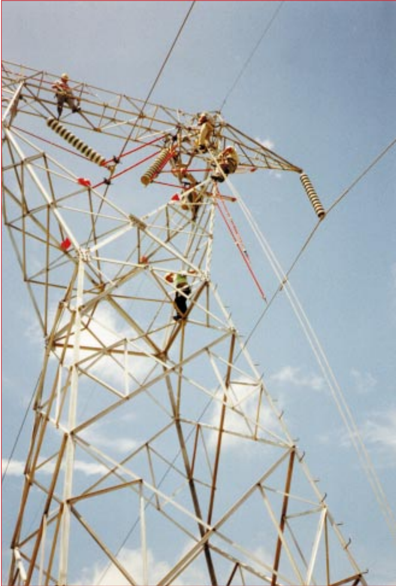
Costa Rica, left, a maintenance crew gets on-the-job training from Chance Hot-Line Tool Specialists atop this 230 kV tower. The V-string of insulators is supported in an Epoxiglas® cradle positioned by wire-tong hot sticks.
