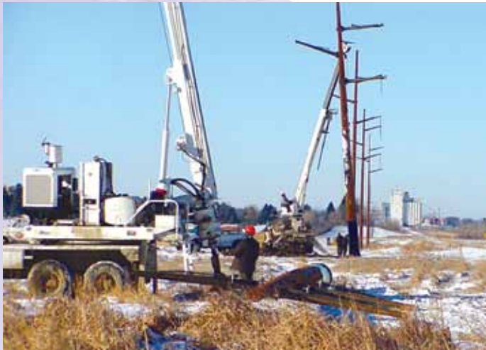
Setting 90-ft weathering steel pole on rerouted 230-kV line, Devils Lake, ND
