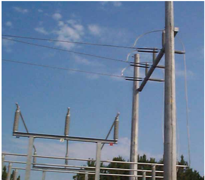
Protecta*Lite is used for all transmission substations. Units are placed in parallel with the string of deadend insulators.
