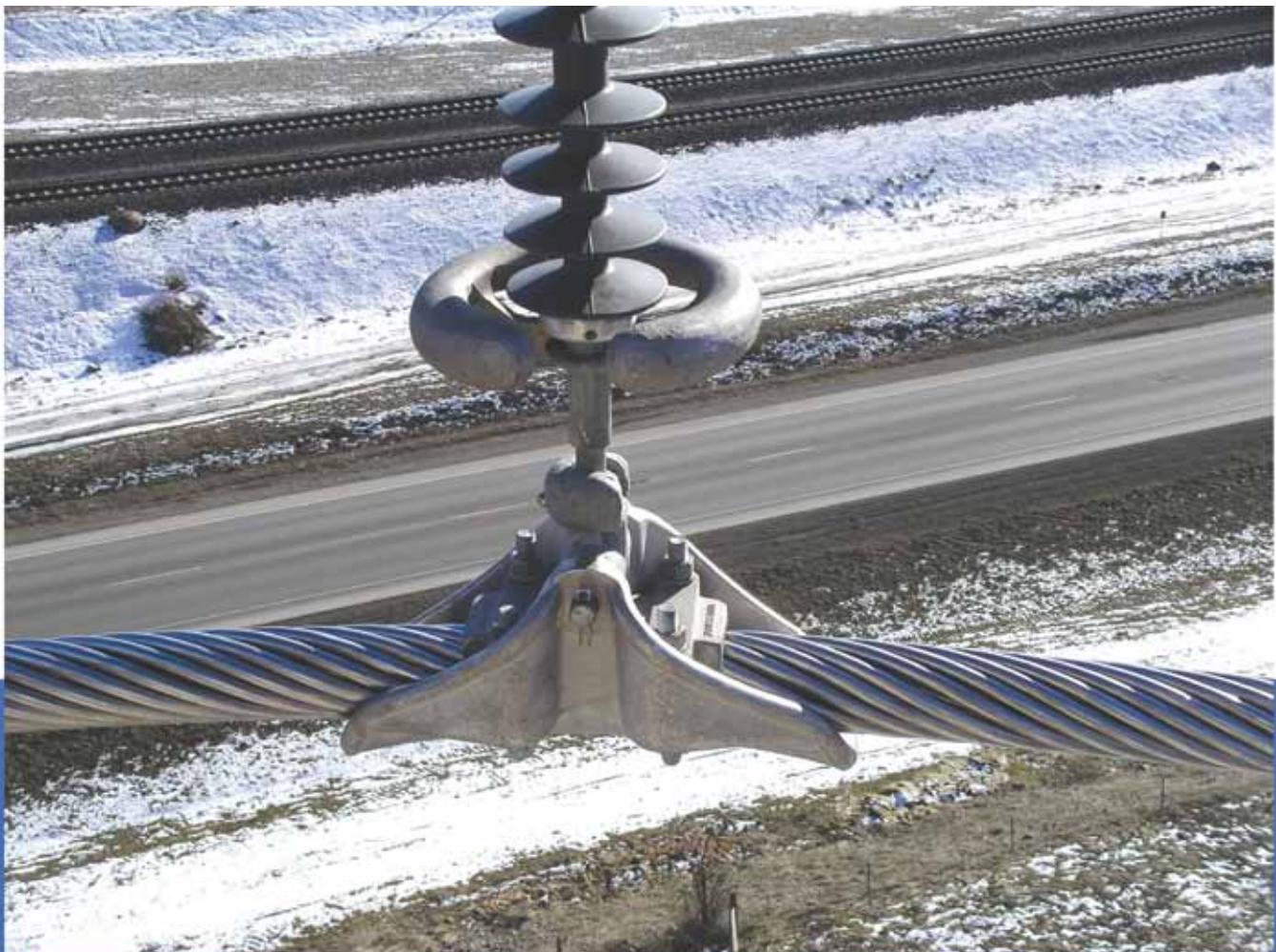
Below: Close-up view of polymer insulator string attached to Anderson ACSS suspension clamp.
