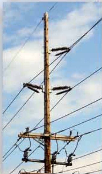
69-kV wood pole structure shows overhead ground wire and PROTECTA*LITE Arresters in parallel with insulators for lightning protection.
