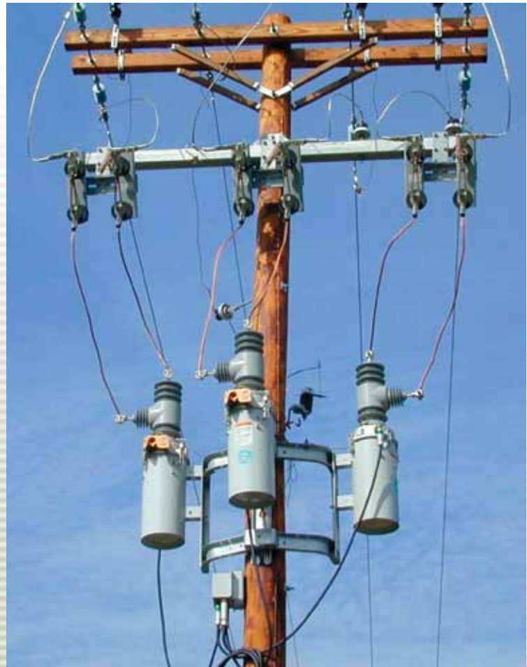
Clean-appearing one-lift installation of three BP3 By-Pass Switches was quick and easy with three-phase mounting bracket configured by Hubbell Power Systems for Harrison REMC.
