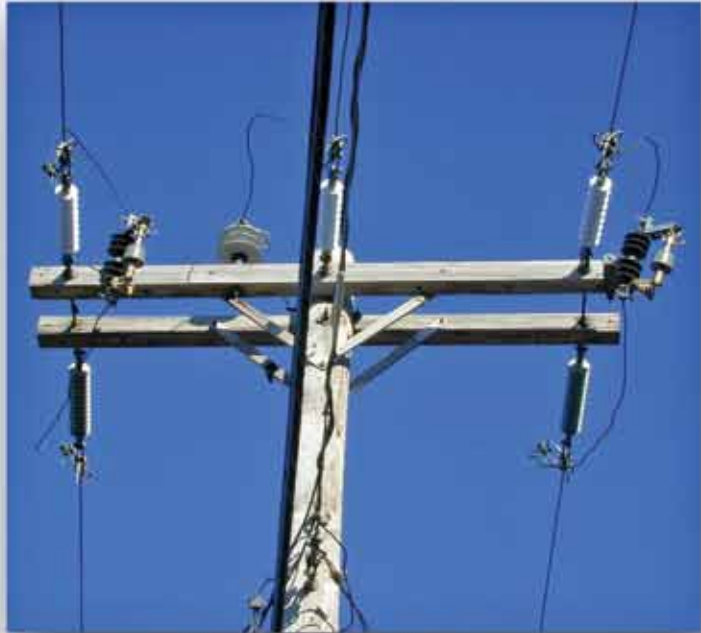
Hubbell electronic sectionalizers fit in a cutout, just as a standard fuseholder, as installed here on the Green Mountain Power Corporation system.
