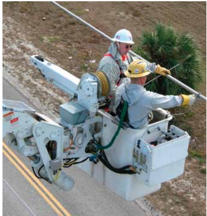
LCEC transmission lineman makes connection to the line with a bonding clamp as instructed by Randy Beckes, Chance Tool Demonstrator.
