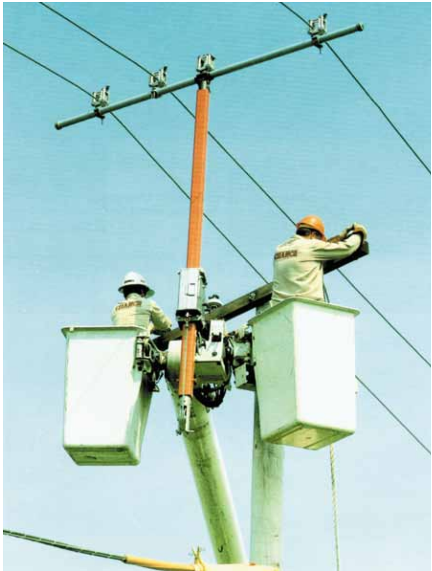
With phase conductors lifted and held at proper clearance, linemen attend to such maintenance tasks as replacing insulators or crossarm.
