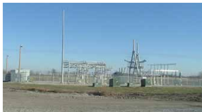
Overall view of Gentry Substation. From left to right: Substation control house, 34.5-kV switch and buss structure, two 34.5-kV breakers, main transformer (34.5/161 kV), 161-kV breaker, 161-kV switch, 161-kV bus, 161-kV transmission line dead-end structure with switches. The tall pole is for lightning protection.
