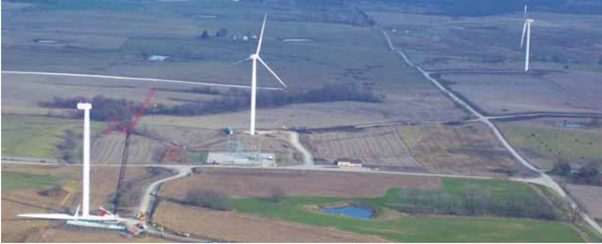
Aerial view of turbines, the main crane for the erection of the turbines, and the Gentry Substation.
